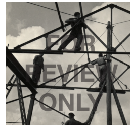
Roman Vishniac Zionist youth learning construction techniques and building new living quarters, Werkdorp Wieringen, The Netherlands, 1939 © Mara Vishniac Kohn Courtesy of the International Center of Photography
